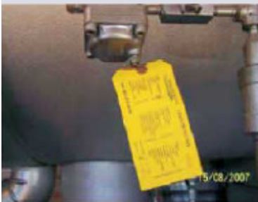
Fugitive emission tagging on the components
