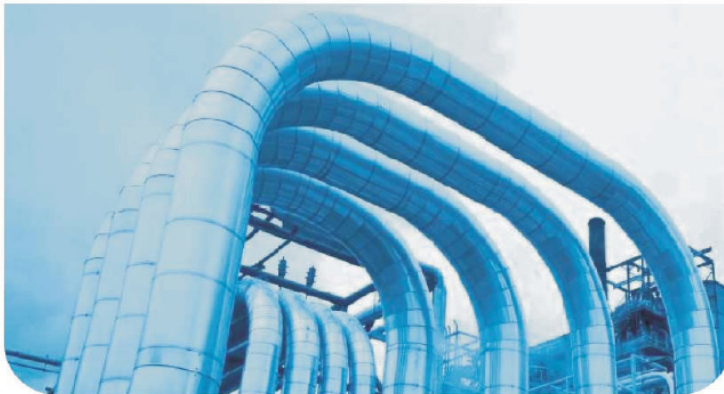
Fugitive natural gas emission management
